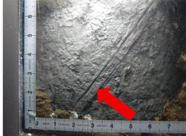
Photo 8: Partial deterioration of the spiral weld at pile 61:D.
