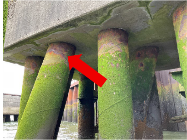
Photo 2: Inshore mooring dolphin, note splash zone corrosion of piles.
