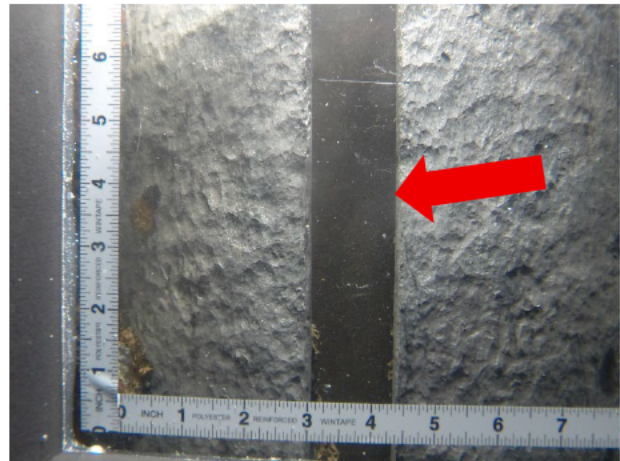
Photo 10: Severe failure of vertical weld seam at Pile 52:B.
