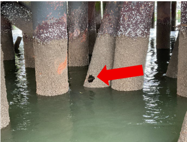
Photo 11: Severe corrosion on Pile 50:B.5, at low water.
